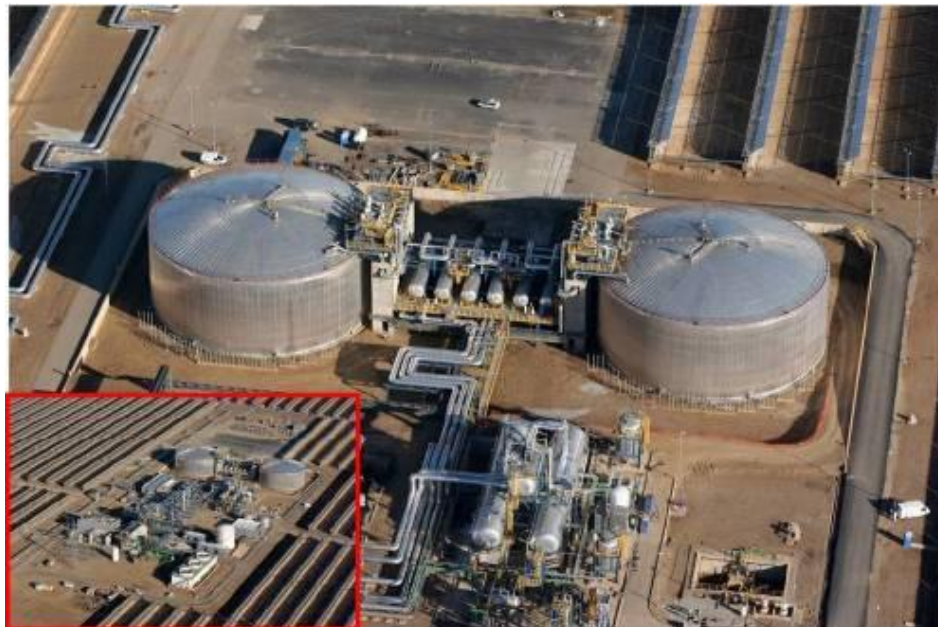
Figure 72 The storage system in the Andasol-1 plant (Relloso, 2009).
